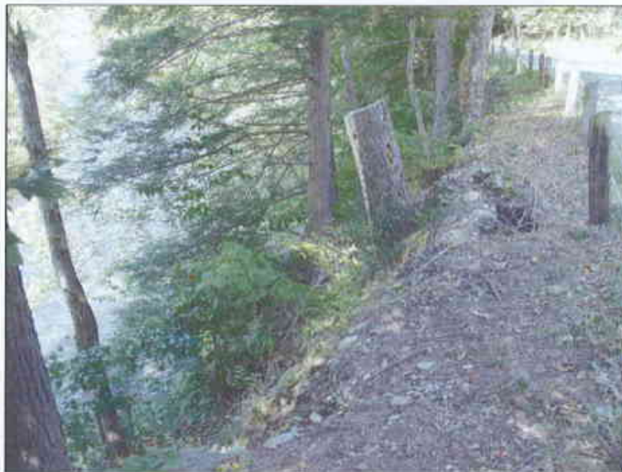
Bank Instability located within Segment 1B on left (east) bank of the West branch
