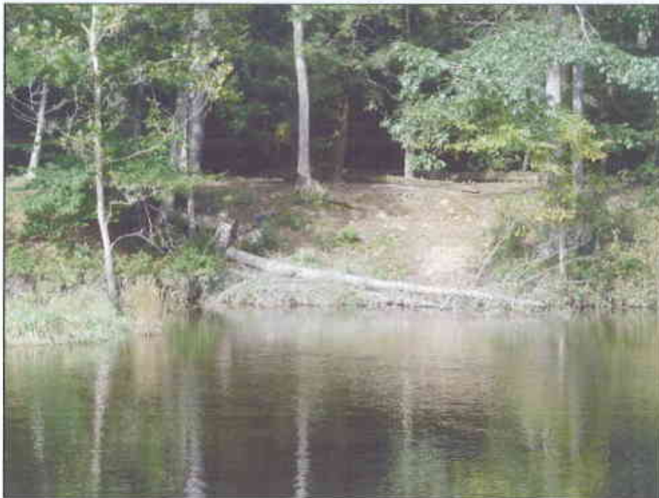
Minor bank erosion located along the left (east) bank within CTDEP State Park.
