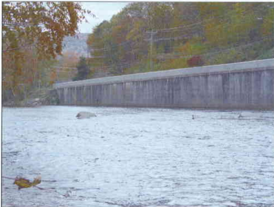
Route 44 retaining wall located along the right (west) bank of West Branch
